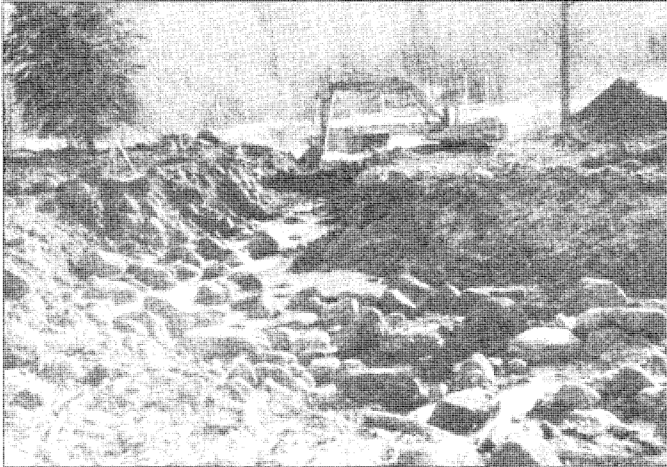
Figure 4-44: Excavation of the first upstream meander bend above the highway bridge in the North Pine project (Figure 4-40 shows the pre-excavation channel).
