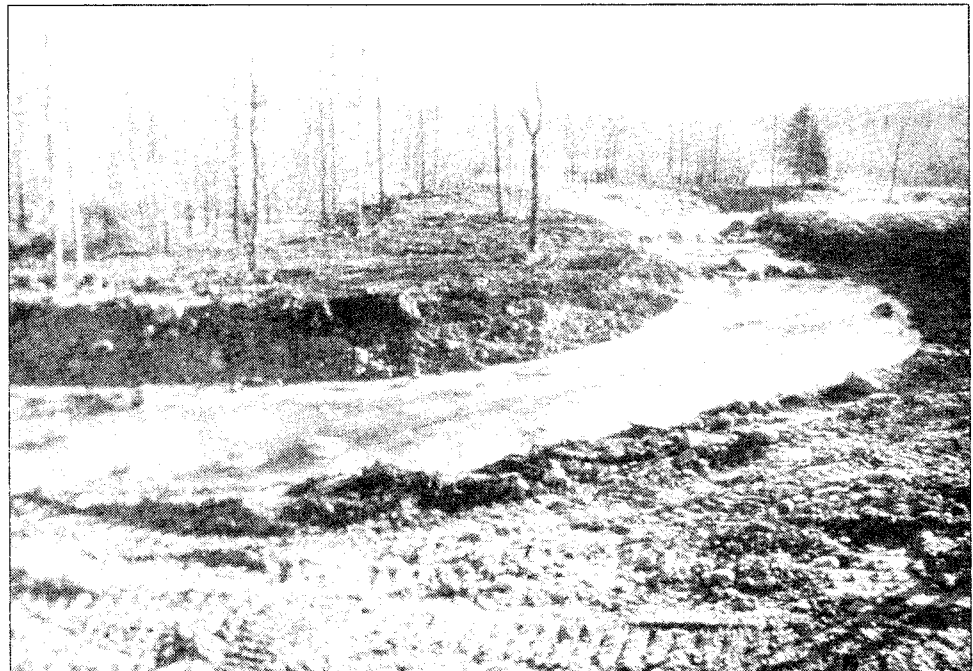
Figure 4-45: The completed upstream meander bend of the North Pine River trout habitat enhancement project (December 1990).
