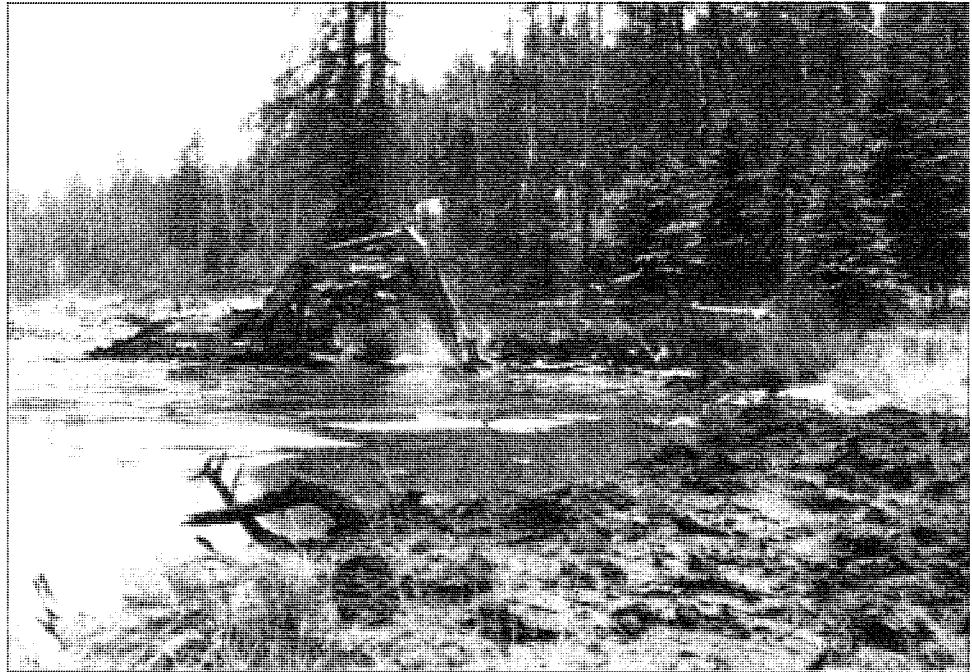
Figure 4-60: Pool excavation prior to constructing cover structure at Station 500. Fill used to re-direct the flow from the original channel is shown in the foreground.
