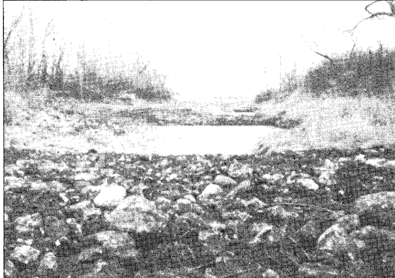
Figure 4-34: Riffle pair on the Wilson River following construction under low flow conditions.
